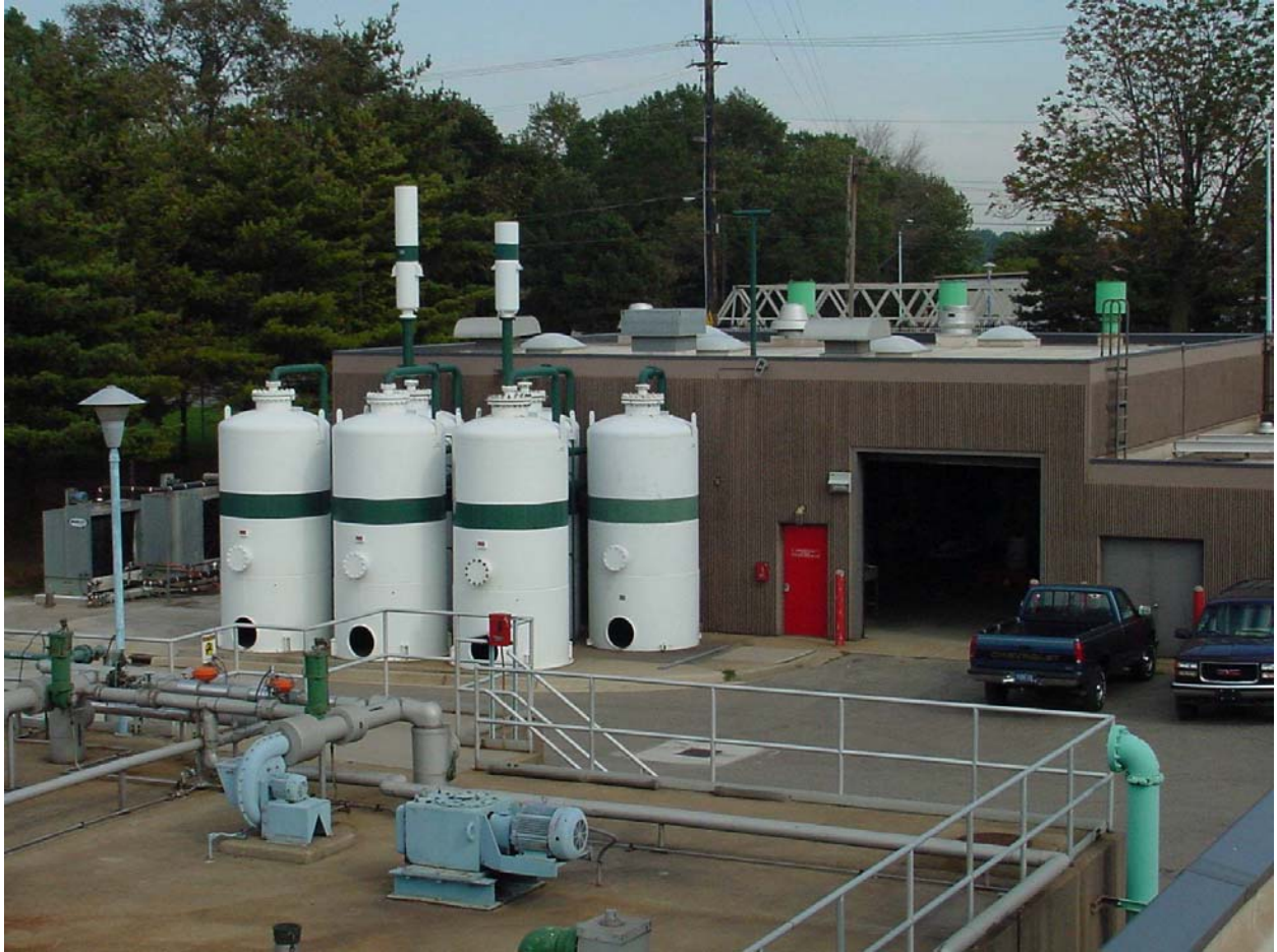
Report prepared by David Ver Hoef, Superintendent WWTP Submitted by David G. Koster, Operations Director
